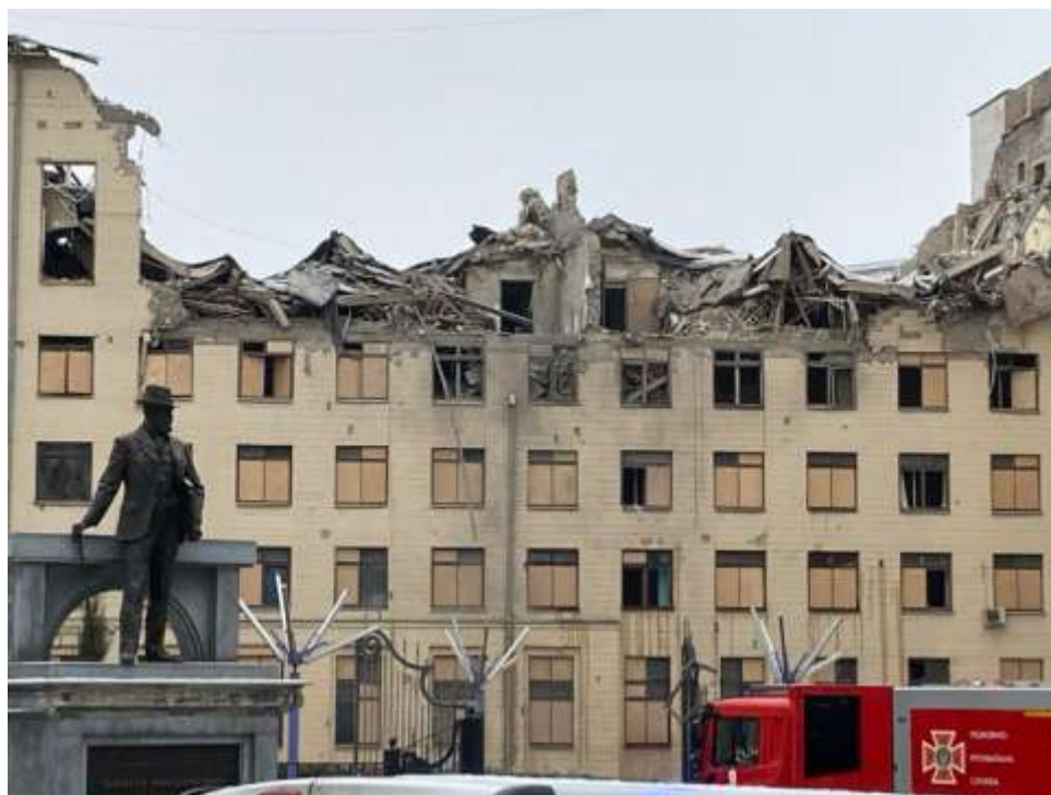
Figure 2: O. M. Beketov National University of Urban Economy in Kharkiv ruined by Russian rocket
